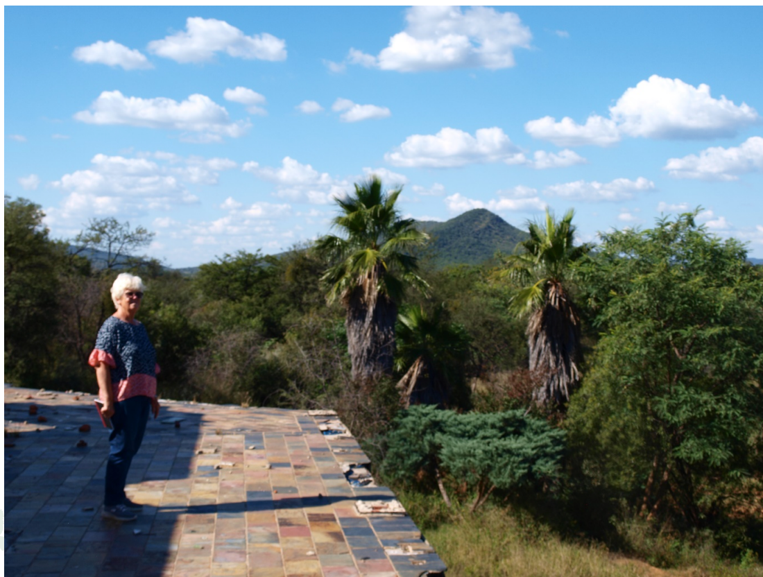
The view from the upstairs deck of the derelict Lobatse Golf Clubhouse
